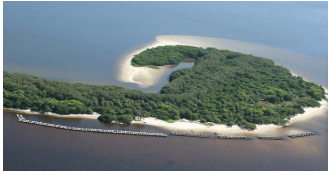
Figure 6. Breakwater installed in 2011 and 2014 along north shore of Sunken Island at Alafia Bank Bird Sanctuary Photo: John Landon, 10/17/14
